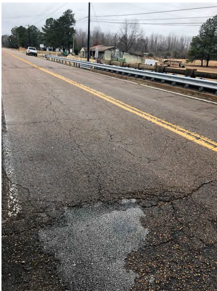
Extensive Pavement Cracking and Rutting on Bridge
