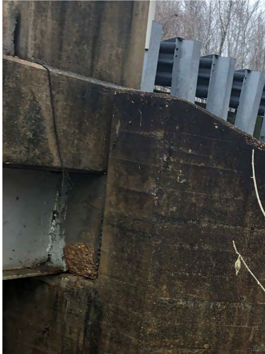
Corrosion and Decay at Girder Connection to East Abutment on Inlet Side
