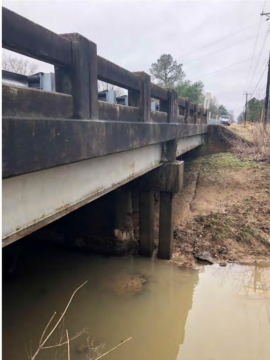
Corrosion on Girder at Outlet
